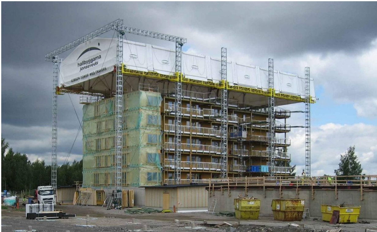
Figure 2. The weather protection system with integrated overhead crane (Photo by J. Vessby, June 2007).
