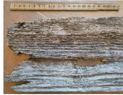
Fig. 2 : A "tavillon" of Alder from the façade on Fig. 1 is showing a nail hole, which has become bigger and where crack formed from it to the edge.
