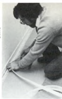
Weatherstripping baseboards and window ledges and installing insulation around electrical sockets are part of an energy retrofit at LeBreton.
