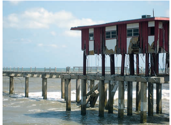
Figure 2. Elevating assets reduces their vulnerability to storm surges, however if the hazard and/or exposure are great enough, the risk may still be large.
