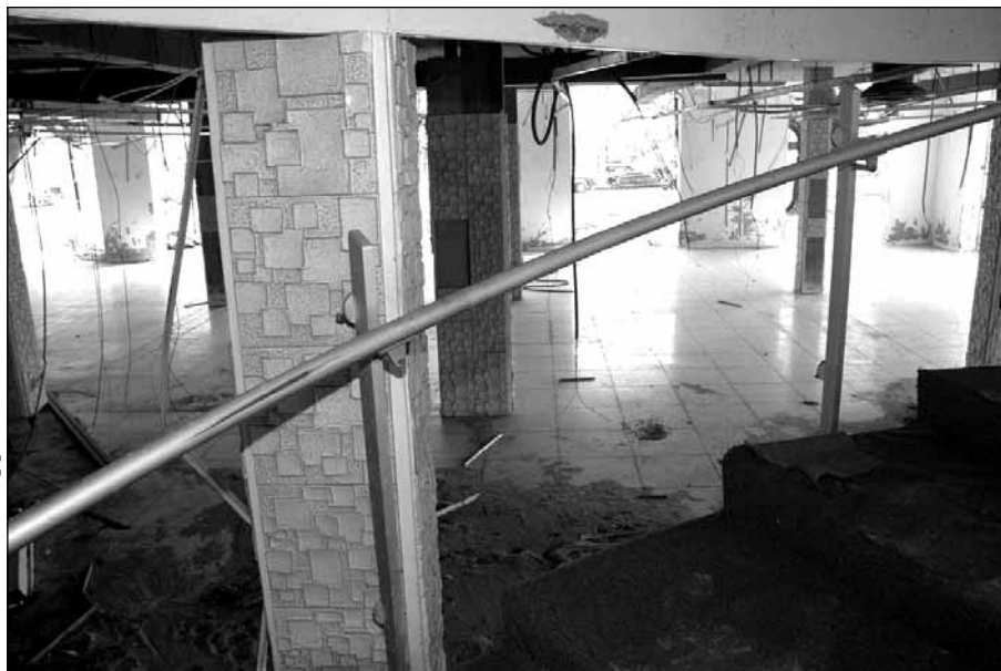
Gulfport-Harrison County Public Library, the ground floor washed out by Hurricane Katrina's storm surge.
