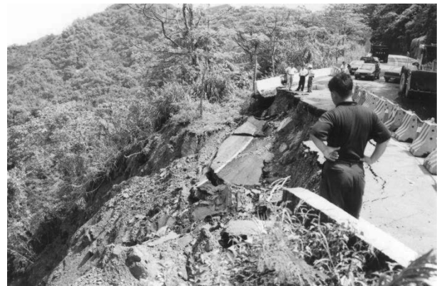
Figure 5. Slope failure at Mileage 39Km due to 2002 monsoon rainfalls.
