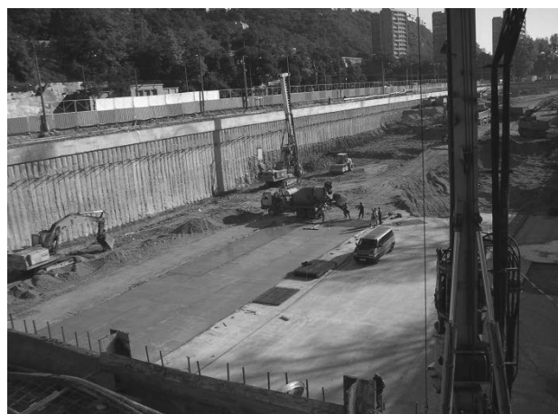
Figure 5. Foundation pit with dimensions of 265 x 53,5 m and depth of 12 m next to Danube river.
