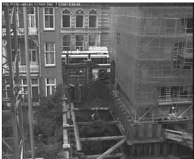
Figure 13. Building pit at PP44 during incident
