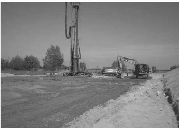
Figure 4. installation of CMC combined with vertical drains and pore-water on the platform
