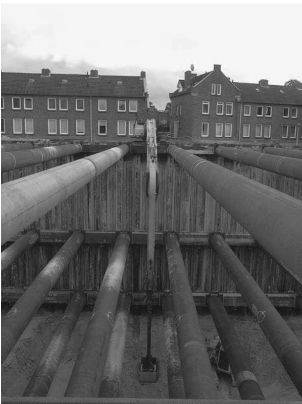
Figure 2. Application of OM in Maastricht for A2Maastricht tunnel (photo Reen van Beek)
