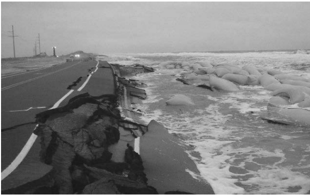
Figure 2. High ocean waves from Hurricane Sandy lap against Highway 12 and erode the underlying sand. (Photo: News & Observer, Nov. 14, 2012)
