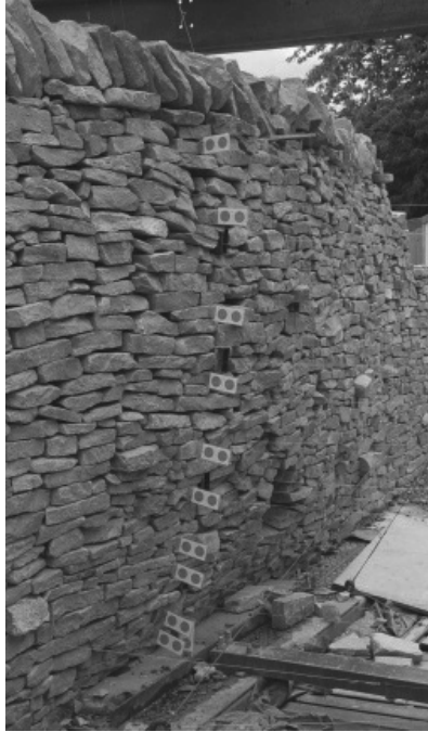
Figure 2. 2.4m high test wall at the University of Bath showing a classic bulged profile in a limestone wall of horizontal construction.
