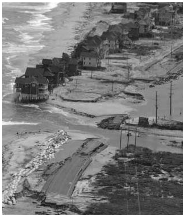
Figure 1. A section of Highway 12 at the edge of Rodanthe, N.C. undermined by erosion due to the storm surge and wave action during Hurricane Irene. (Photo: News & Observer, Aug. 31, 2011)
