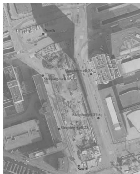
Figure 7. Positioning of the four ‘sleeping’ wells east and west of the building pit. Additional wells may be installed at the north and south side in case of a calamity in the northern or southern wall.
