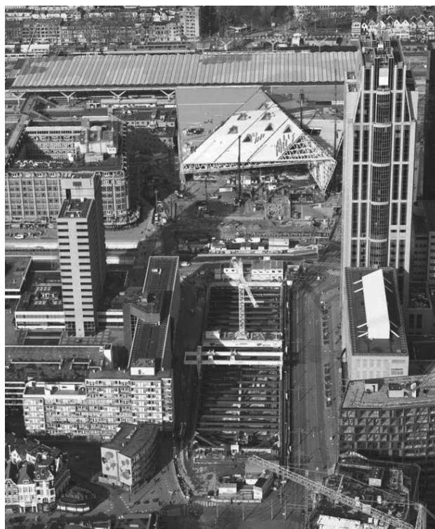
Figure 1. The construction of the underground car park Kruisplein (February 2012). The apartment building is situated in front, at the left (perpendicular to the car park). Photograph Nick de Jonge – Skeyes fotografie.
