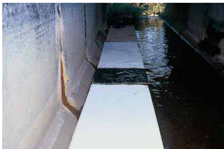
Figure 9 : Ledge for small animals in culvert with ink-method (Photo by H. Bekker)
