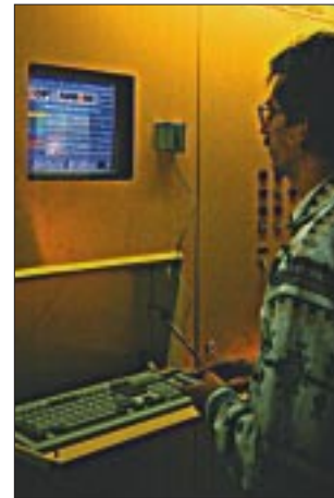
At the co-generation plant, a monitor and an optional keyboard are the entrance to the entire expert system.
